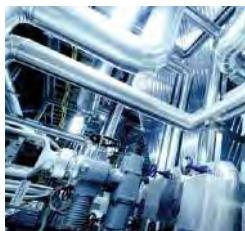
Typical high-corrosive environment — central utility plants.
